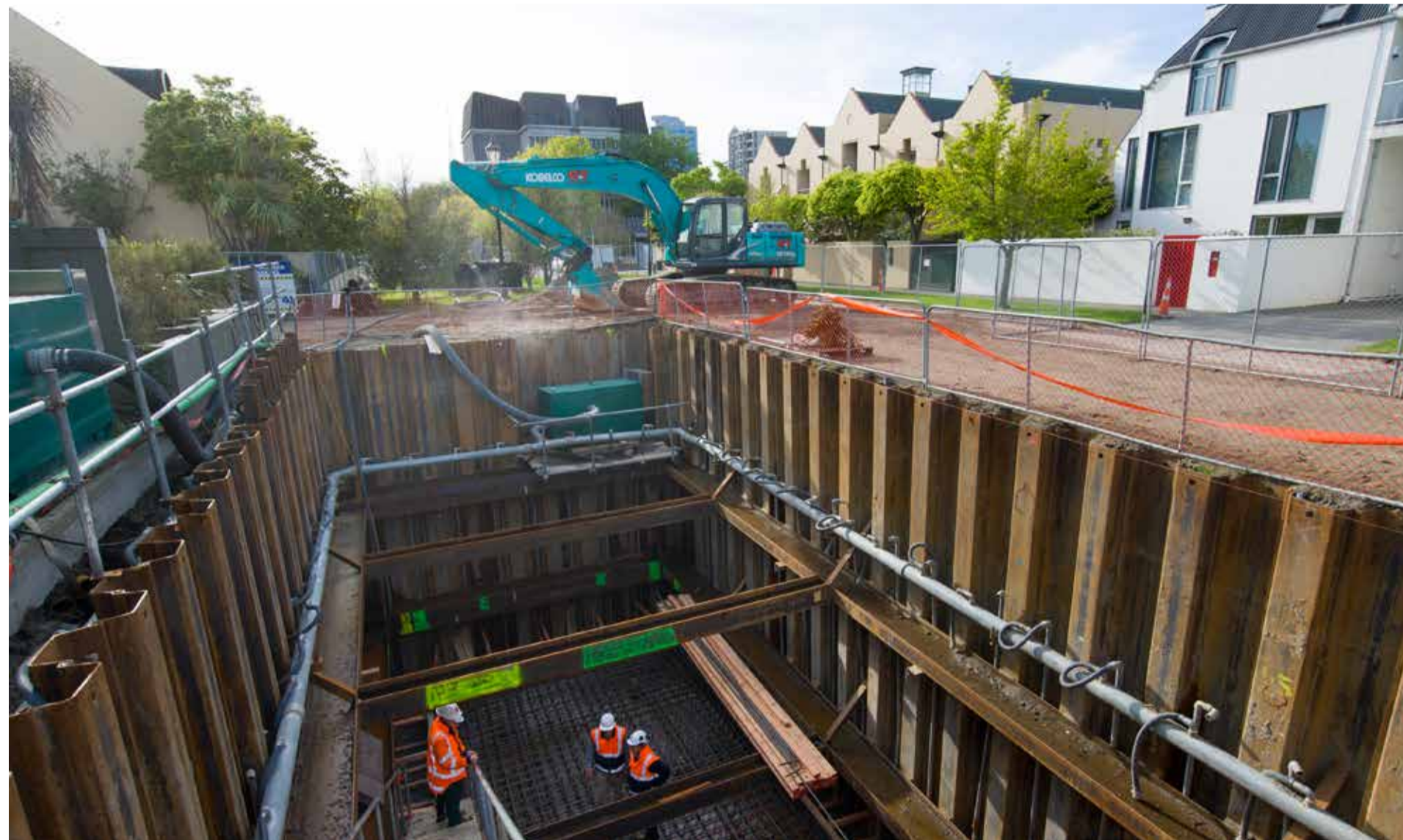
SCIRT excavated a very large trench in Chester Street West in 2013 for the installation of the central city's largest underground pump station.
