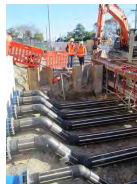
Six vacuum arms in a new pump station on Bexley Reserve suck wastewater from households in Aranui to the pump station.
