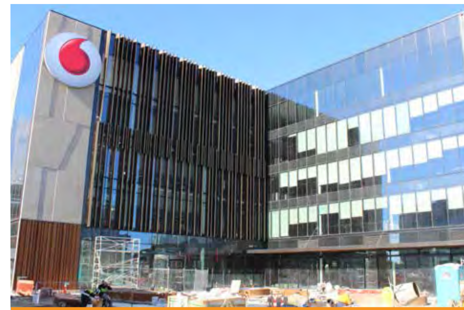
Work is underway on landscaped public spaces (shown here behind the new Vodafone building) that will continue throughout the South Frame.
