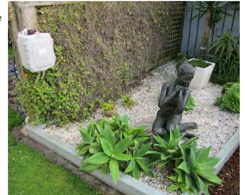
A pressure tank installed underground in a private property. Only the lid and an alert panel on the fence are visible.
