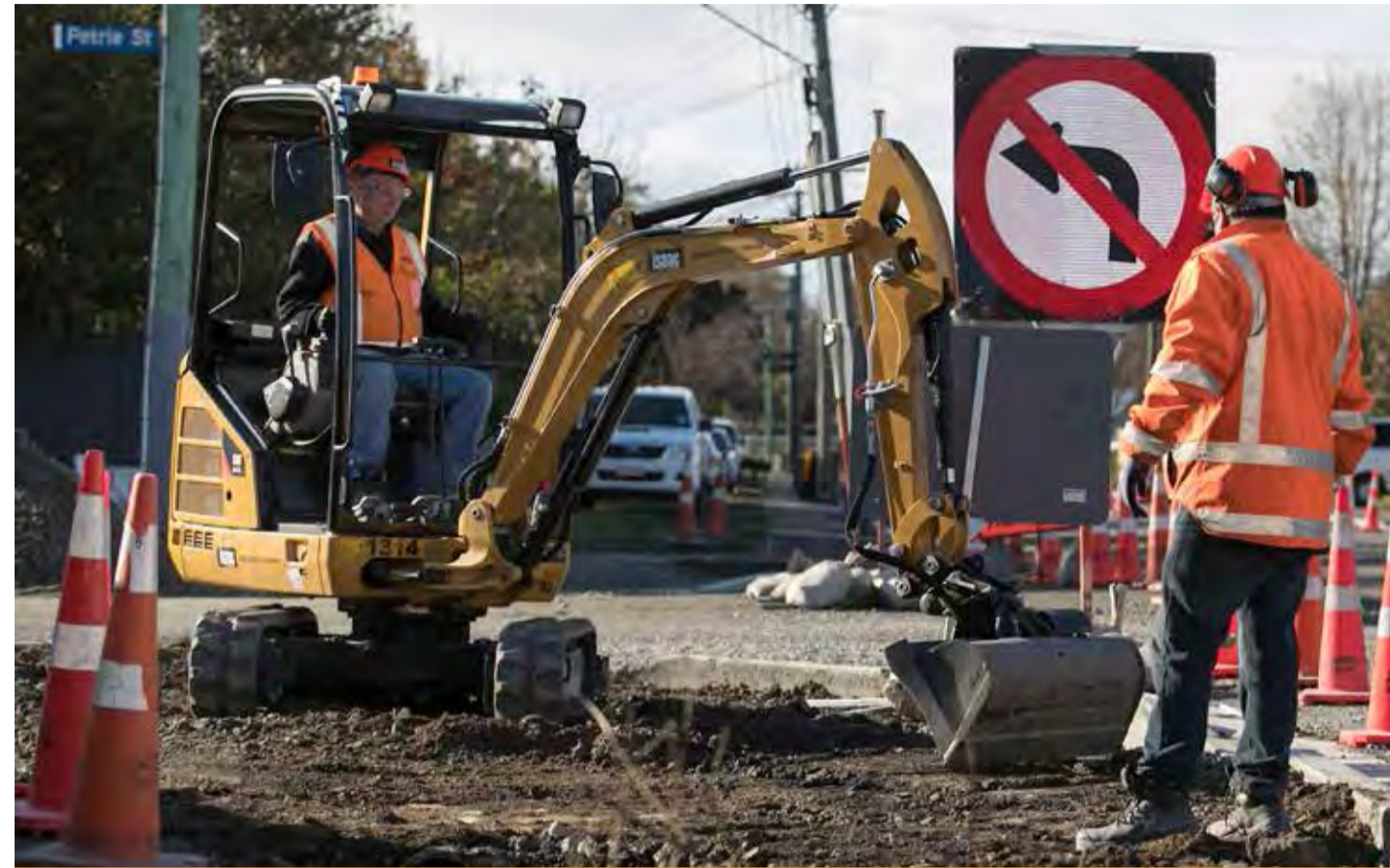
Contractors dig out the footpath as part of the Petrie Street repairs in Richmond.
