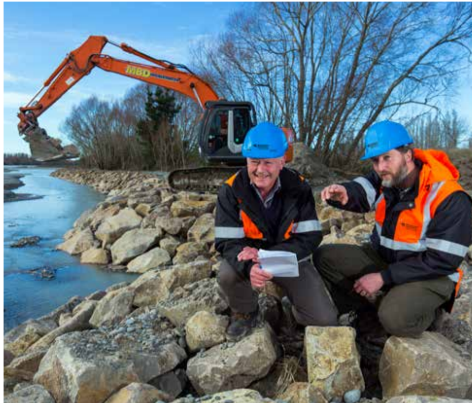
Environment Canterbury Principal River Engineer and Project Leader Ian Heslop (left, photographed with colleague Matthew Surman) says the Waimakariri Flood Protection Project will significantly lower the risk of break-out during a major flood.
