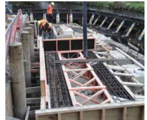
Pipes allowing water to flow through the eel (in Māori, tuna) habitats are installed during construction.
